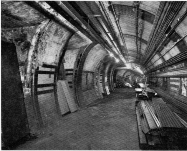
Lower lift landing for the mainline station entrance, closed 1968. Photo Nick Catford
